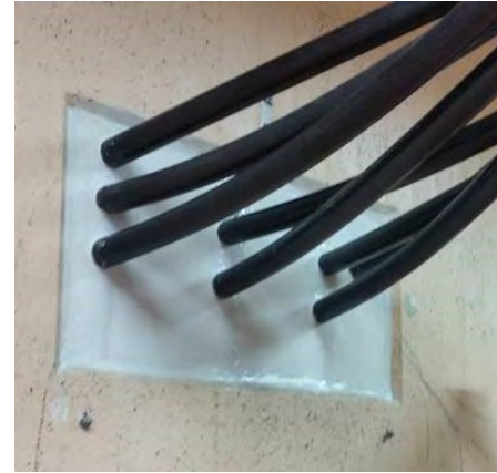
Typical sample of penetrating services with gaps above 30mm or mixed services
