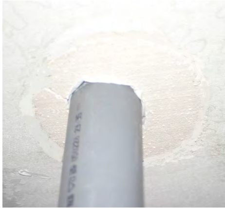
Typical sample of penetrating services with gap widths between 0 and 10mm
