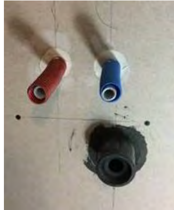
Typical sample of penetrating services with gap widths between 10 and 30mm
